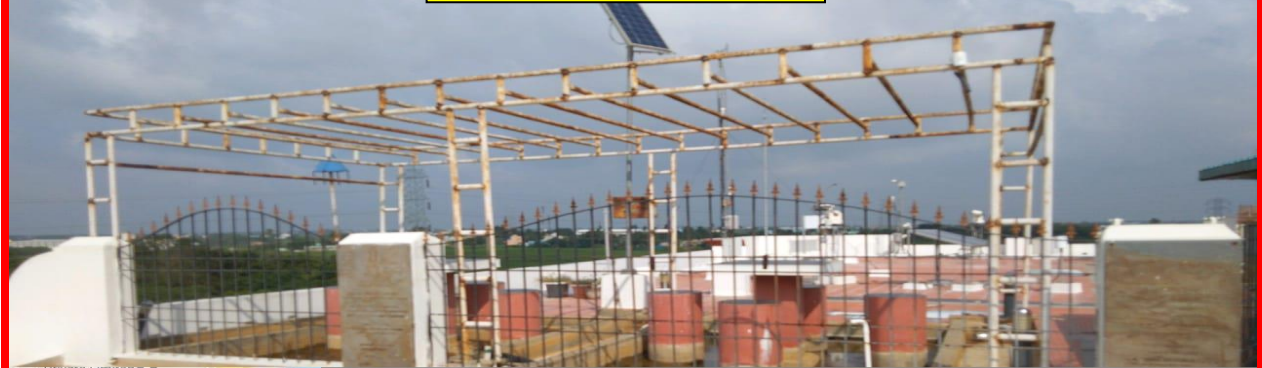
Solar plant at main block
