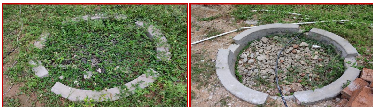
Fig.2: Rain Water Harvesting Pits located in each Buildings
